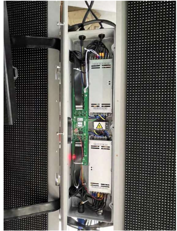
Inside of Power Box
